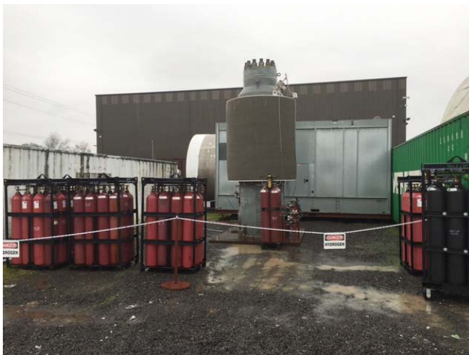
FIGURE 1. Arrangement of the testing site for hydrogen cyclic testing of the demonstration SCCV
