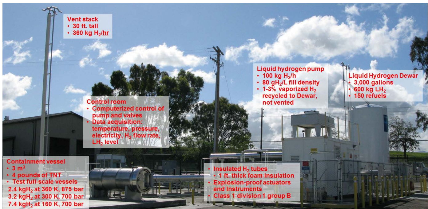
FIGURE 1. Hydrogen test facility at LLNL showing the main components and their performance metrics: liquid hydrogen pump, liquid hydrogen dewar, containment vessel, control room, insulated hydrogen tubes, and vent stack.
