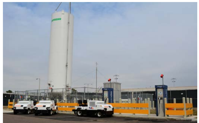
FIGURE 3. Liquid hydrogen station on airport ramp
