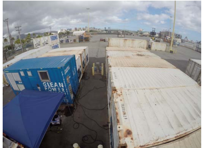
FIGURE 1. The Maritime Fuel Cell Generator (blue container, middle left) contains 75 kg of compressed hydrogen storage and produces over 100 kW net electricity, packaged in a 20-ft shipping container. Here it powers refrigerated containers at Young Brothers, Ltd. in Honolulu Harbor.
