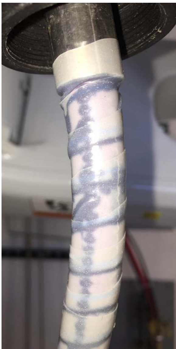
FIGURE 4. Chemochromic leak indication tape on nozzle-side hose end
