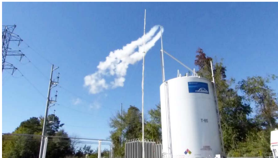
FIGURE 3. The NREL Hydrogen Plume Analyzer deployed during a planned LH2 venting process. The observation of hydrogen below the horizontal release point facilitated the recommendation proposed for future editions of NFPA 2 that the vent stack be designed to direct the release up away from ground level.
