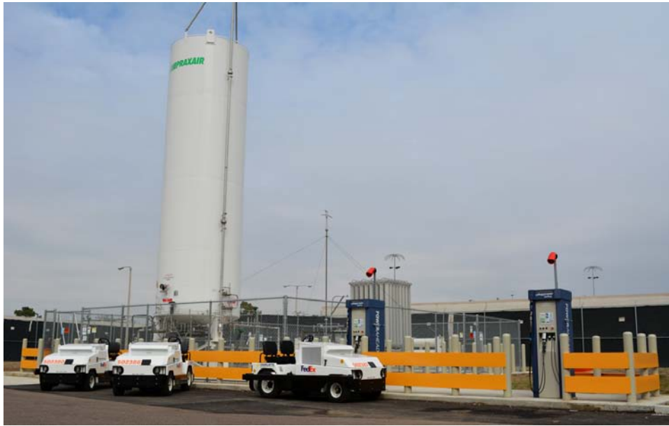
FIGURE 3. Liquid hydrogen station on airport ramp
