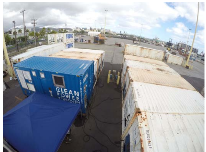
FIGURE 2. The generator (blue) in the “Icehouse” area powering reefers (white)
