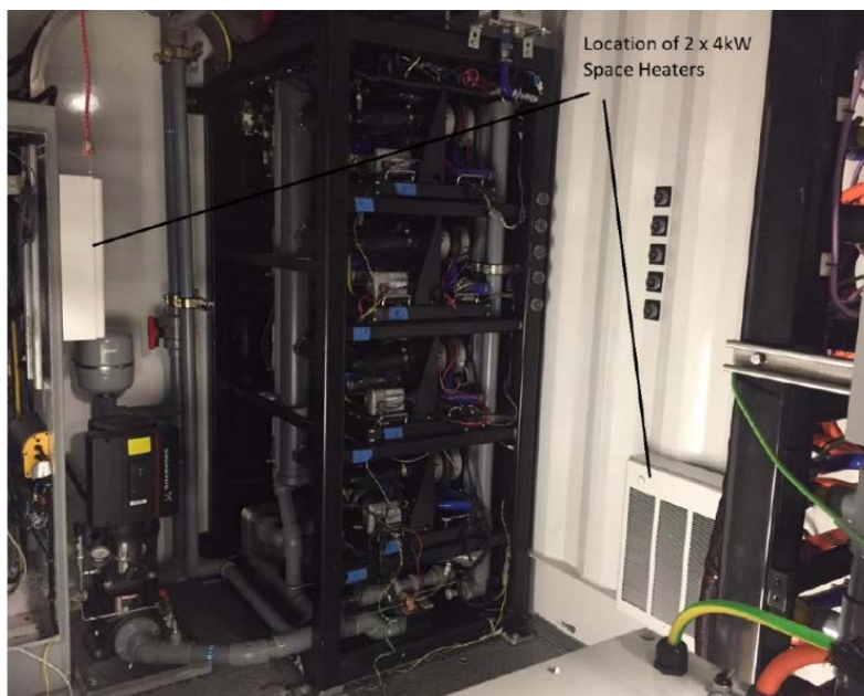
Figure 3. System heaters and controls that were installed to allow the MarFC to operate in weather down to -25^{\circ}\text{C} in anticipation of a future deployment in cold weather
