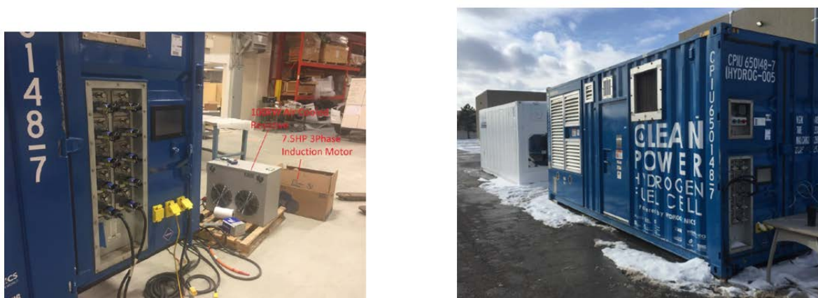
Figure 4. (L) Indoor testing of the MarFC unit at Hydrogenics after system repair and upgrade; (R) outdoor testing of the MarFC unit in cold weather at the Hydrogenics site in Mississauga, Ontario, Canada, December 2017
