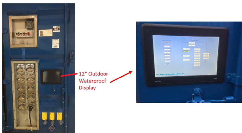
Figure 2. Installation of a ruggedized system display, making it easy for the operator to ascertain the state of the MarFC, especially during start-up
