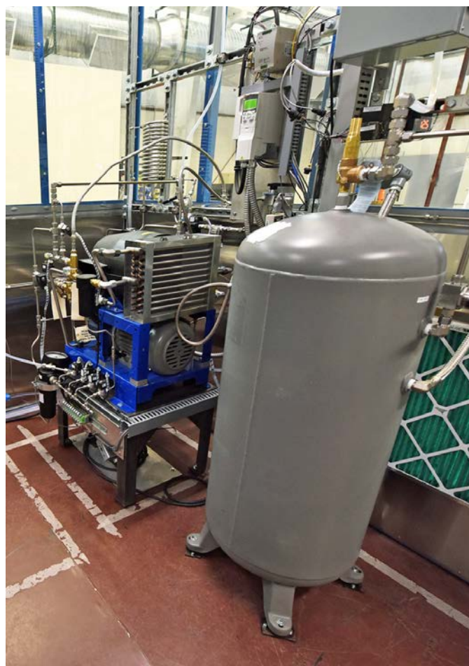
Figure 4. Hydrogen recycle compressors system compressor, storage tank, and counterflow heat exchanger
