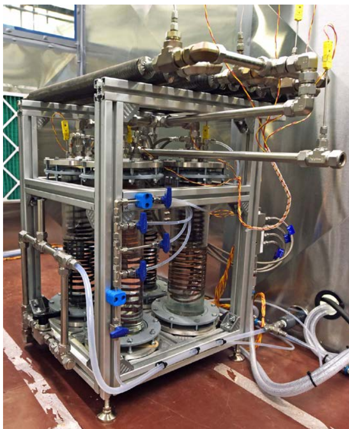
Figure 3. Finned-tube steam coolers and water-cooled condensers
