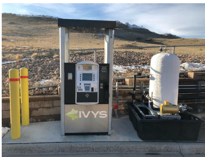
Figure 1. Dispenser and hydrogen cooling system installed at NREL's HITRF
