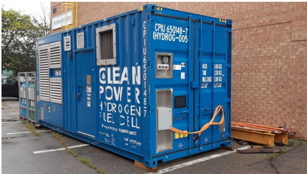
Figure 5. The 100-kW MarFC unit in place for electrical testing at Hydrogenics
