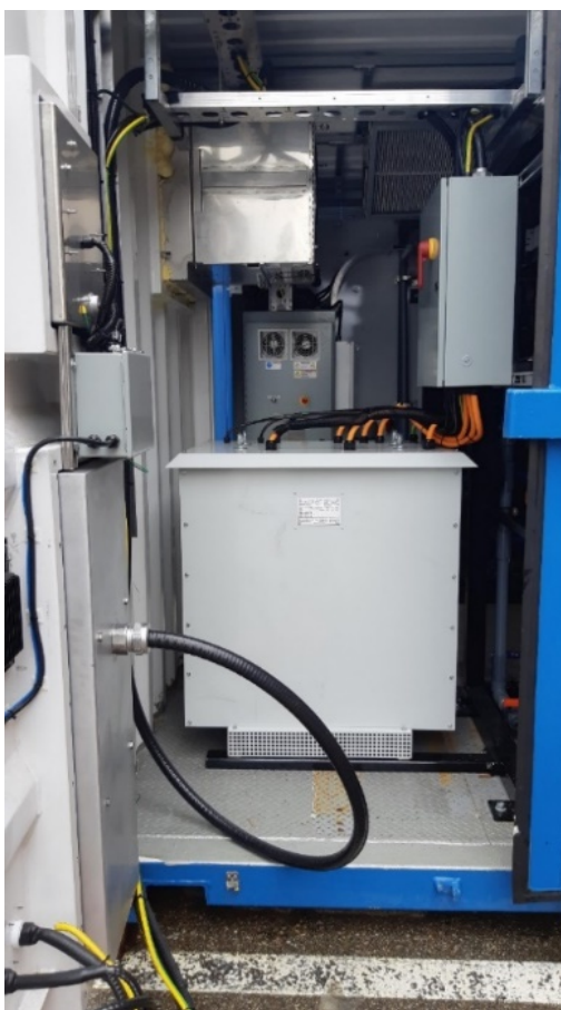
Figure 1. New transformer installed
