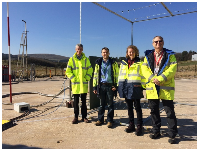
Figure 4. The HSE-NREL team installing the NREL HyWAM at the HSE LH2 release apparatus. (L-R: Simon Coldrick/HSE, Jonathan Hall/HSE, Tashi Wischmeyer/NREL, and William Buttner/NREL)
