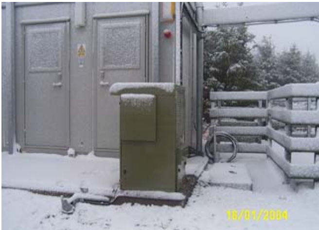
Site Host's Cell Tower
