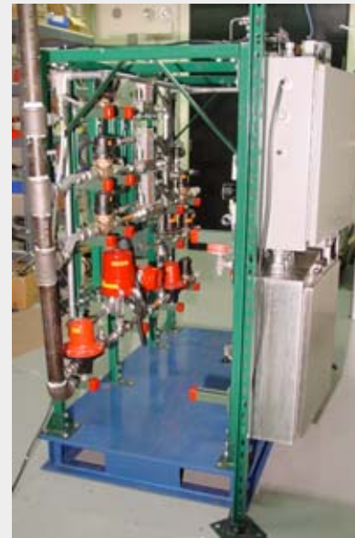
H 2 Generator Controls
