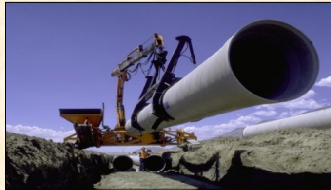
Picture provided courtesy of Ameron International.
