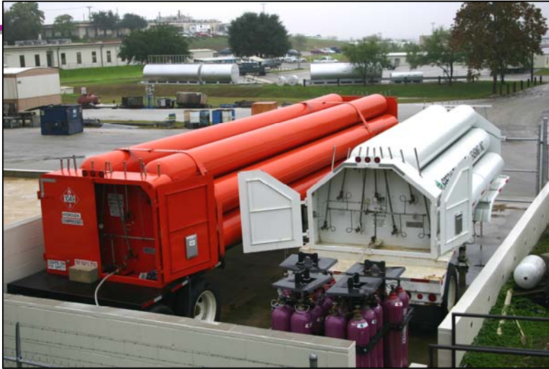
H 2 and He Tube Trailers (Revetment)
