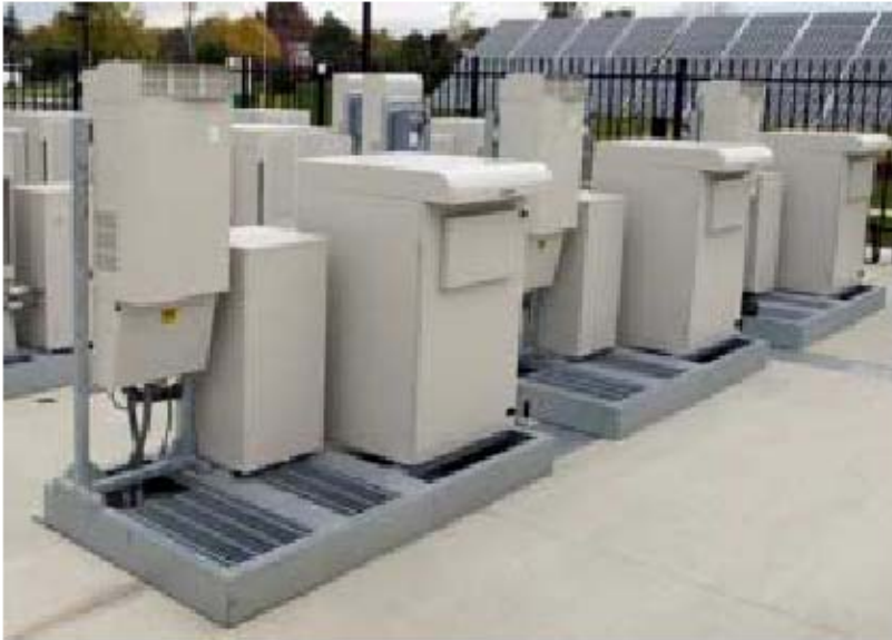
Fuel Cell Power System (50kW)
