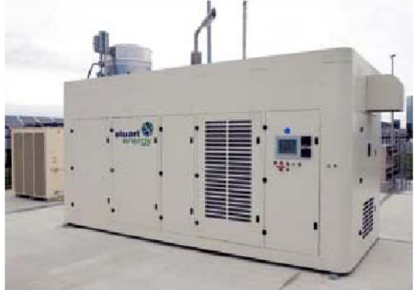
Electrolyzer (2.7kg/hr @ 5700psig)
