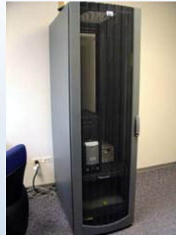
Server, workstation, tape backup and UPS
