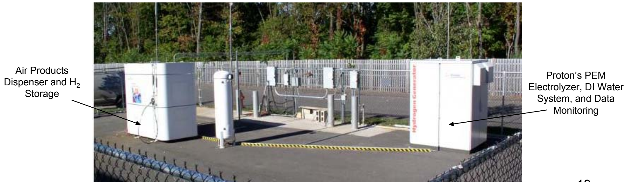
Hydrogen Fueling Station Installed at Proton Energy Systems (Wallingford, CT)
