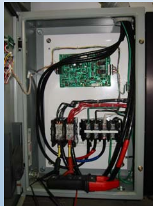
AC-DC Power Electronics
