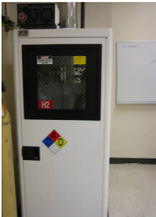
H 2 cylinder cabinet
