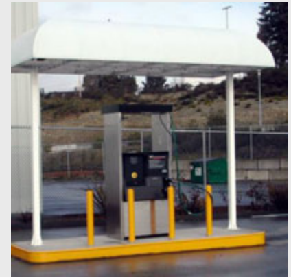
GTI/GreenField H2 dispenser at Victoria, Vancouver Island, BC
