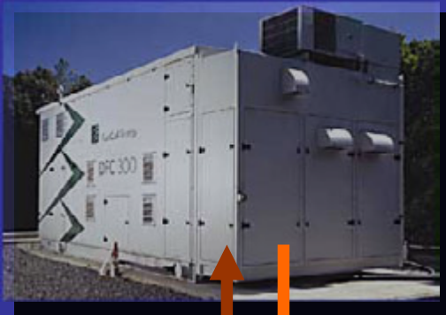
FuelCell Energy DFC-300
