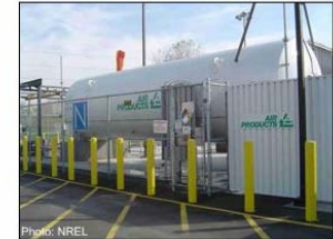
Photo: NREL Liquid hydrogen is stored at Santa Clara Valley Transit Authority (CA), which operates fuel cell buses
