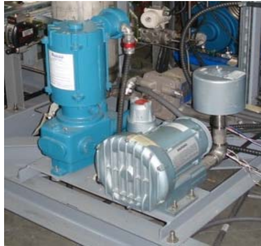
Water pump and air blower
