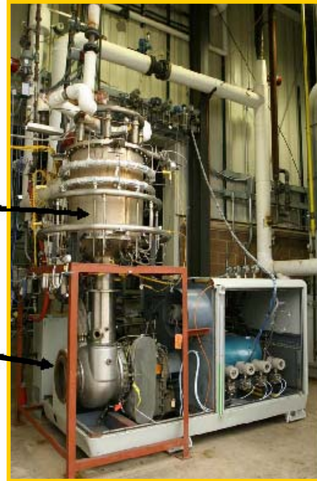
Partial Oxidation Gas Turbine (POGT)
