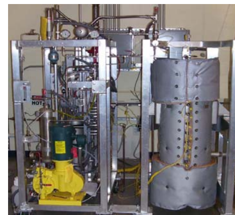
10 kg/day Hydrogen Pilot Plant
