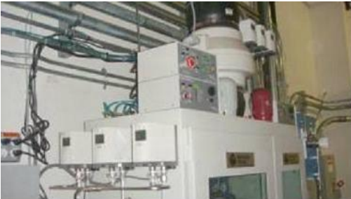
Controlled and Monitored Gas Delivery
