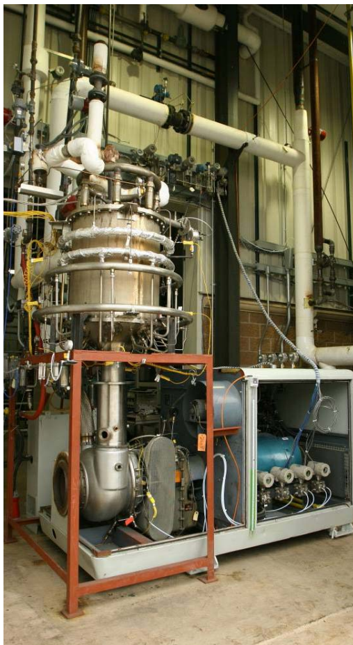
Partial Oxidation Gas Turbine (POGT) & Reactor
