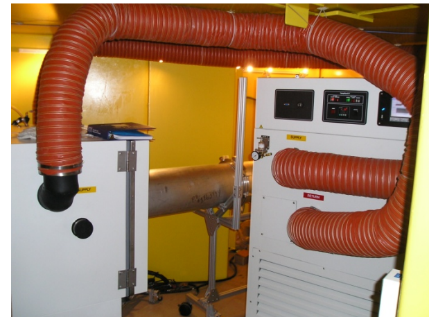
Freeze Chamber Installed inside the Imaging Facility
