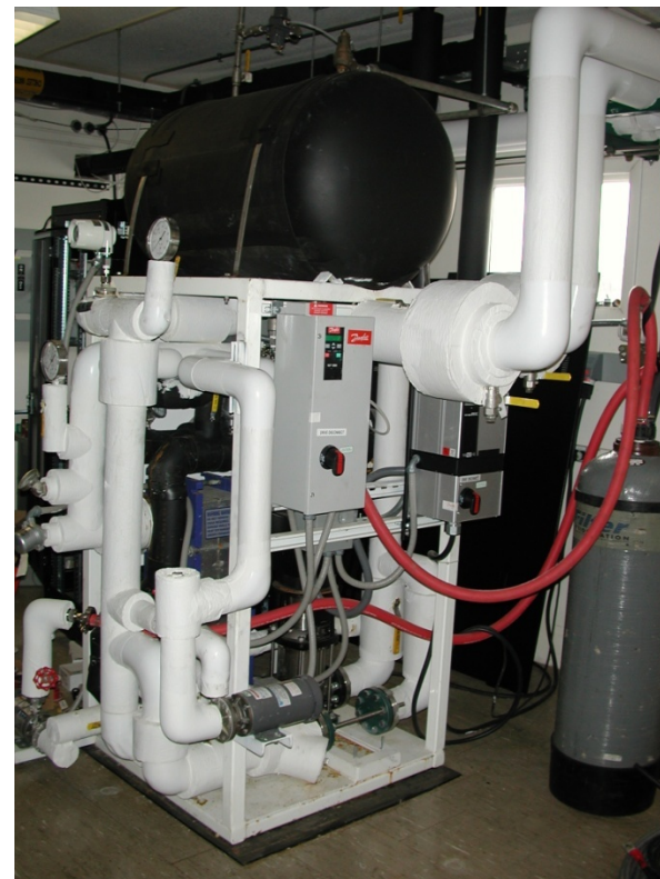
100-kW cooling system installed in the Fuel Cell Test Facility
