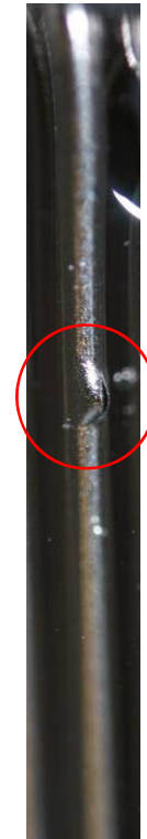
Single tube failure
