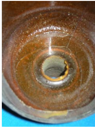
cracks in 3" liner
