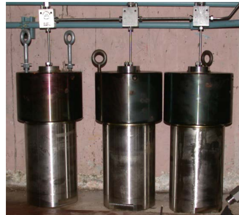
High pressure hydrogen accumulators
