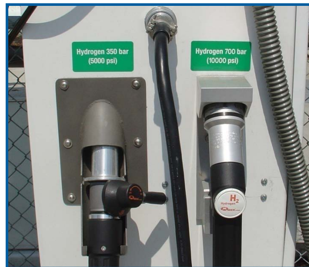
Burbank, CA station. Photo: NREL
