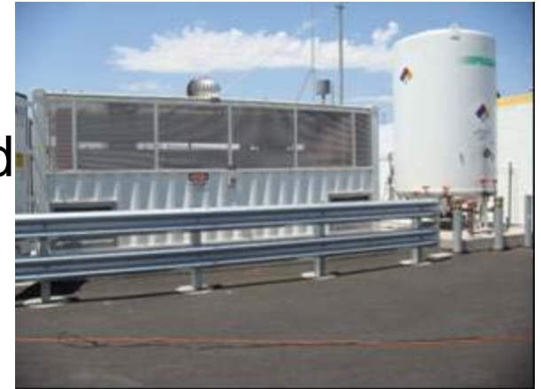
Hydrogen Compression Skid, Culver City, CA
