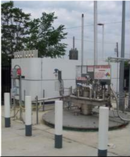
Below-grade LH2 storage, Benning Rd, WDC
