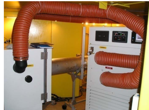
Freeze Chamber Installed inside the Imaging Facility
