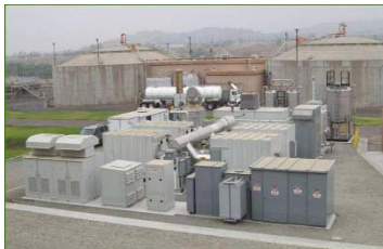
California WWT Plant BioGas CHP
