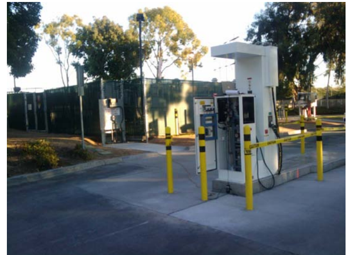
Hydrogen Fueling Station
