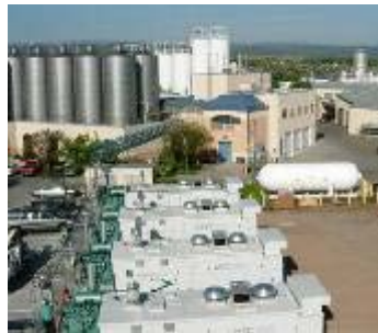
Sierra Nevada Brewery Nat Gas and BioGas CHP
