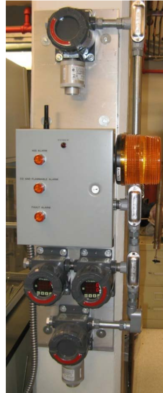
Alarm System in a PNNL Laboratory
