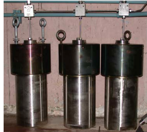
High pressure hydrogen accumulators
