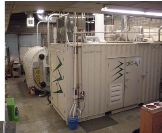
Mechanical Balance of Plant (MBOP)
