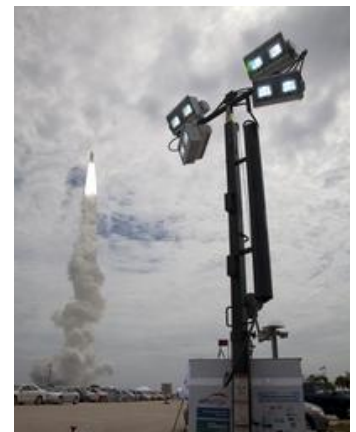
Hydrogen fuel cell powered light tower at Space Shuttle launch
