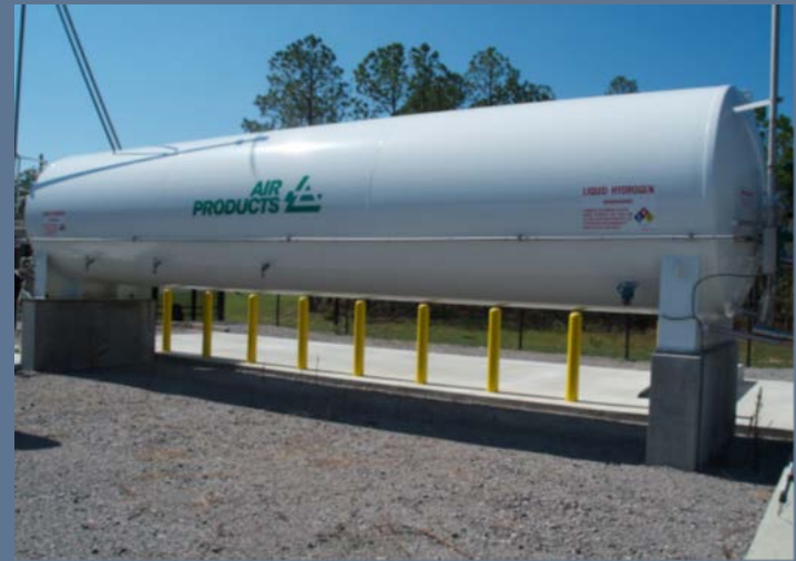
Existing 9000 Gallon Liquid Hydrogen Storage Tank
