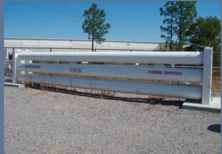
Existing Gaseous Hydrogen Storage Vessels
