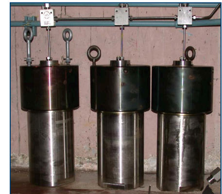
High pressure hydrogen accumulators
