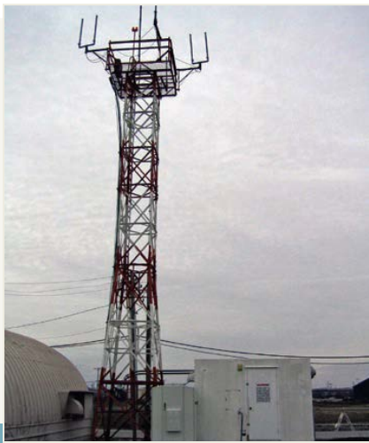
A 1-kW fuel cell system providing power for this FAA radio tower near Chicago
