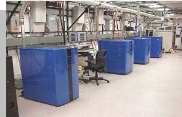
Plug Power Systems Lab
