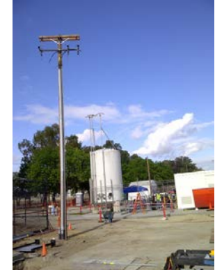
200 m overhead power line
