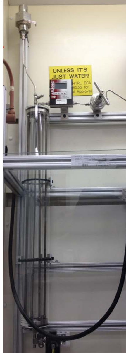
Hydrogen Separator Tank
