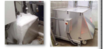
Figure 4. Cold Block and Chiller enable H70 Fast Fill
